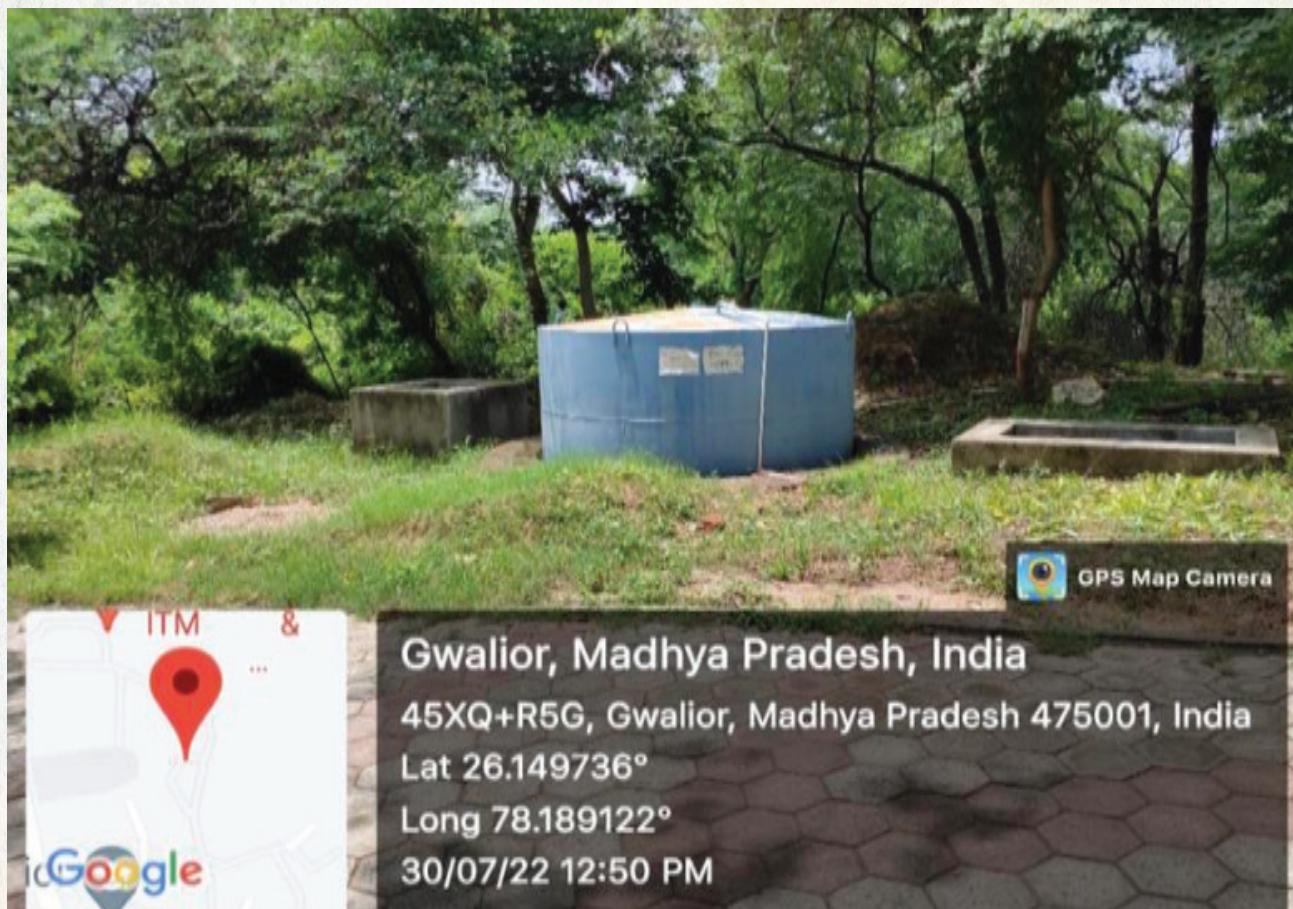
Photos of Bio Gas Plant
