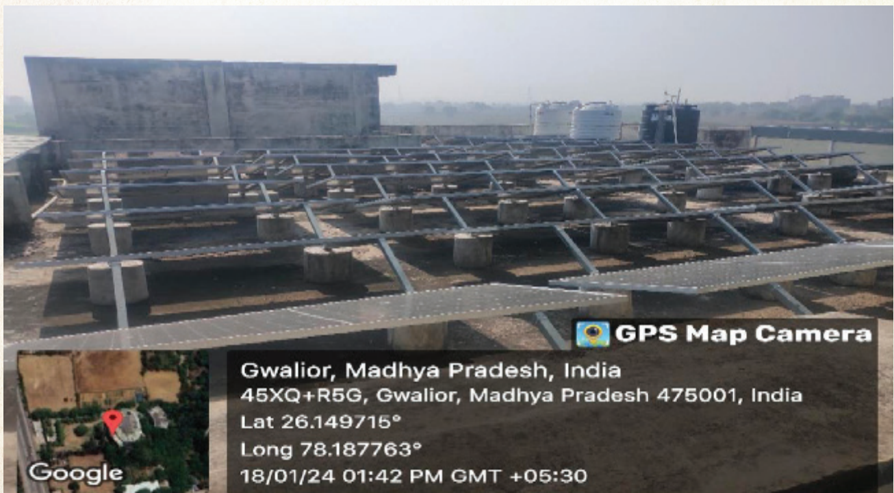
Photos of Solar panels on the roofs of JC Bose Block building
