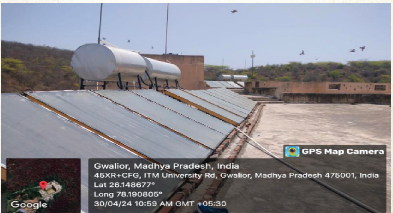
Solar water heating panels on hostel and residential complex
