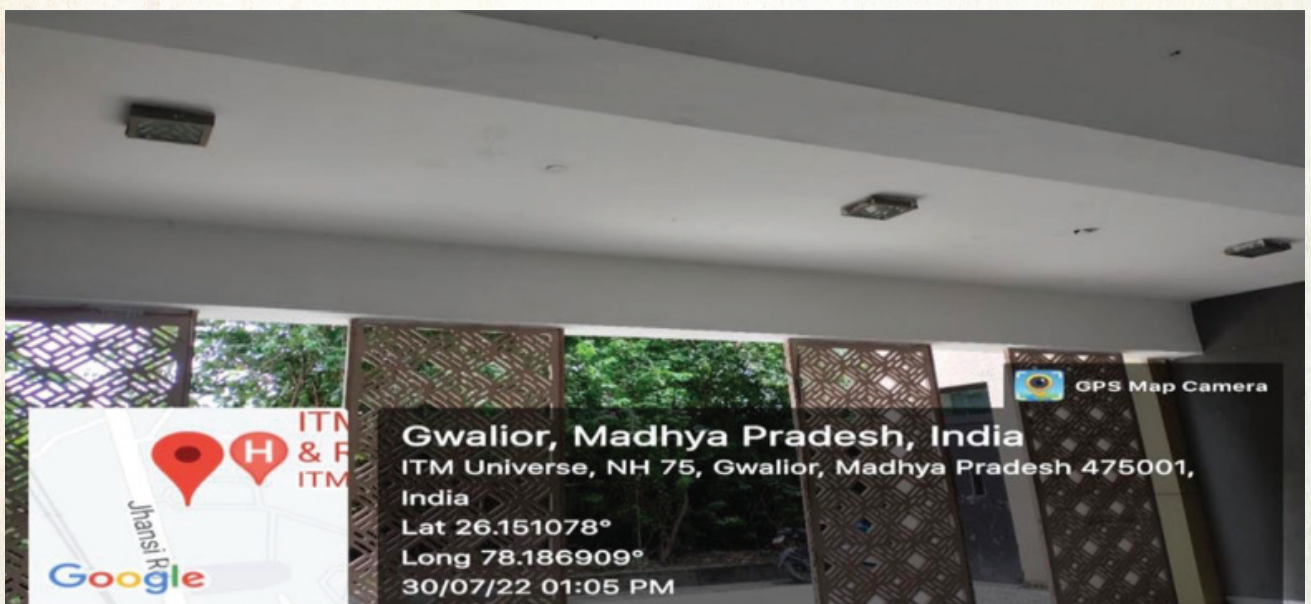
Installed LED BULBS at various Blocks
